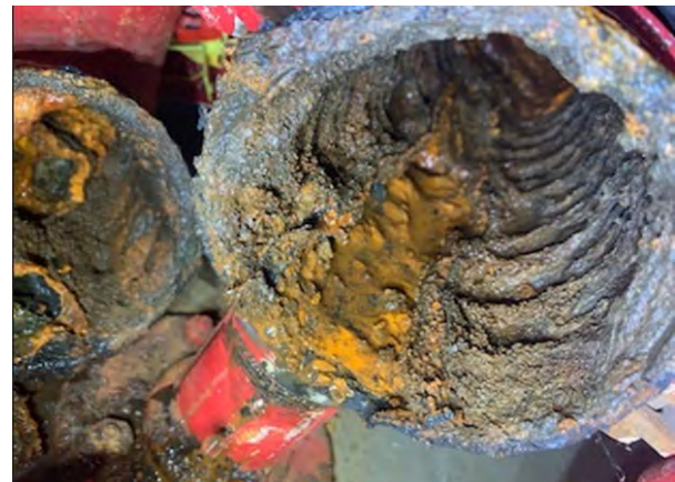
Figure 23. Degraded 222-S Laboratory firewater riser.
