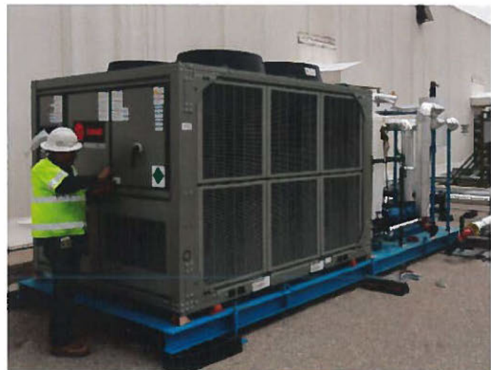
A 40-ton chiller provides supplemental cooling for the RNS drums inside the PermaCon.
