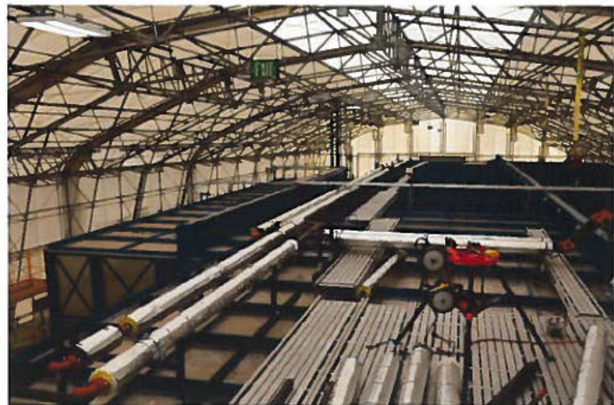
A supplemental cooling system was installed where the RNS drums are stored.
