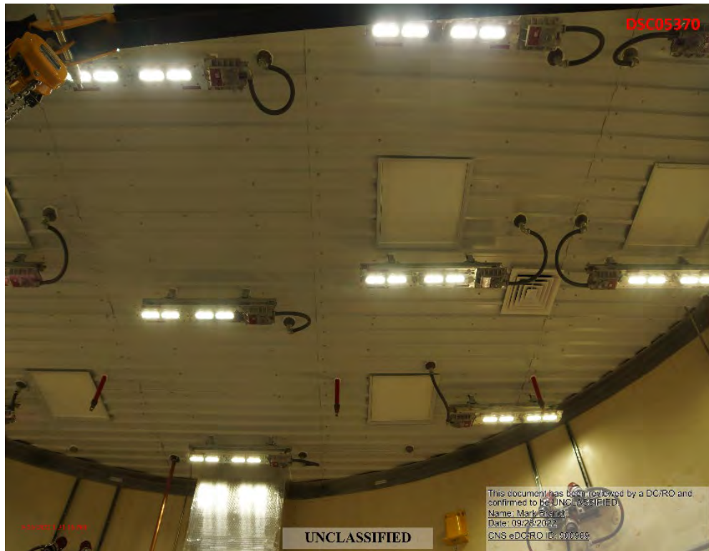
Figure 1. Upgraded False Ceiling within a 12-44 Nuclear Explosive Cell
